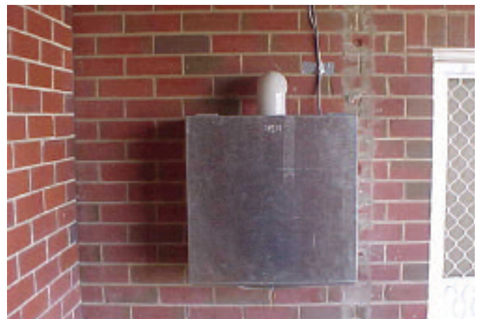
Figure 1: E-nose installed in an outside location at a meat works
