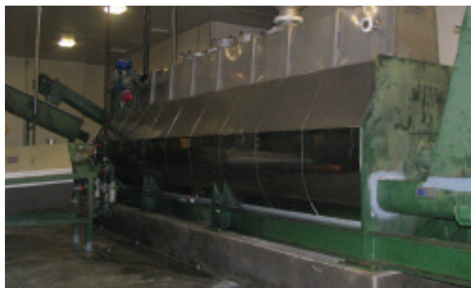
Figure 3: All rendering processes in Australia must be tested annually to show that the heat treatment can eliminate C. perfringens
