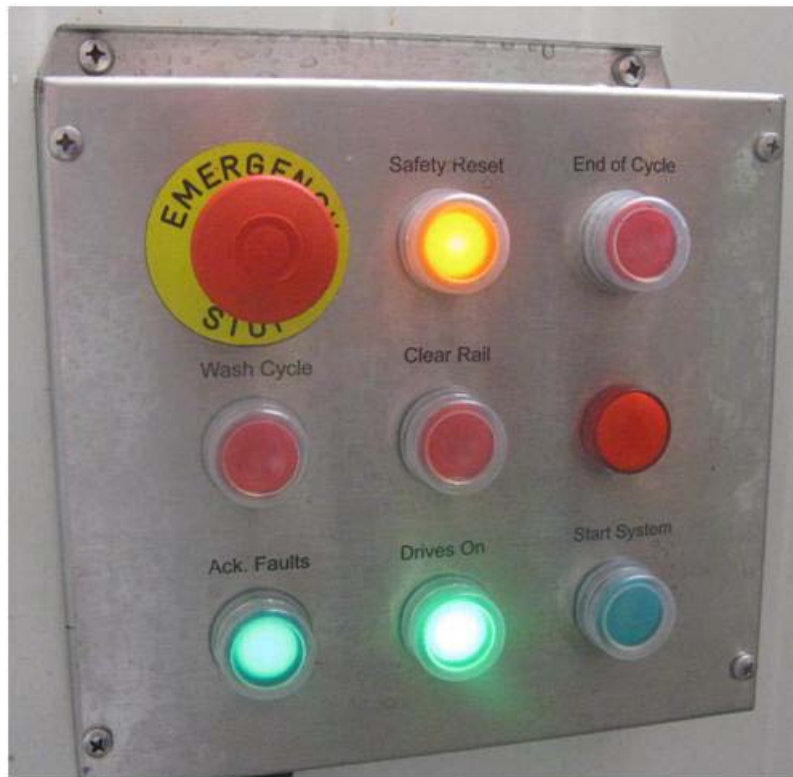
Figure 7: Operators panel used to operate the equipment.
