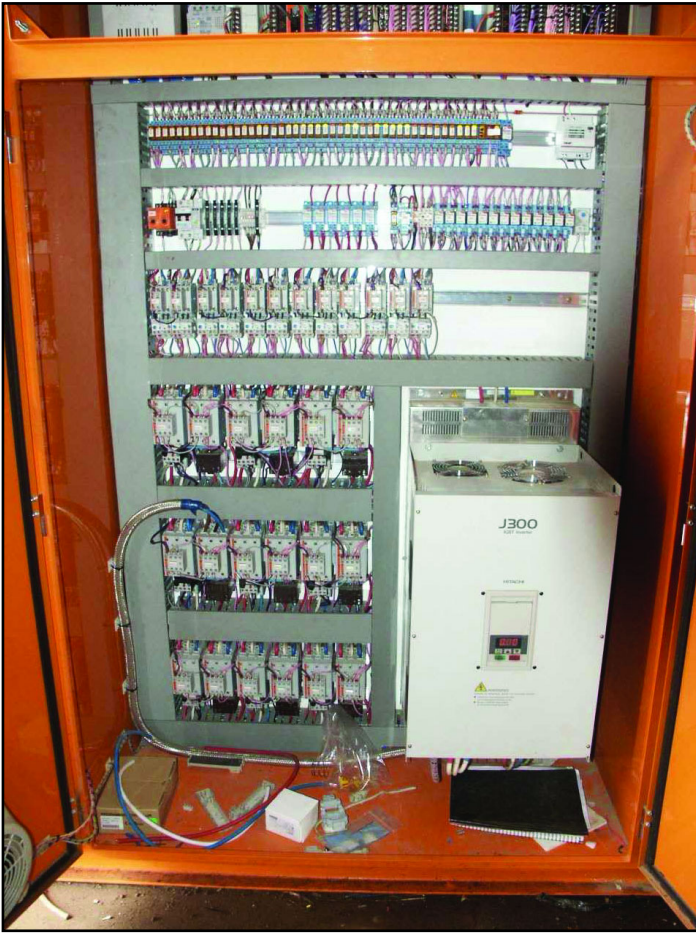
Photograph 1: Refrigeration control panel
