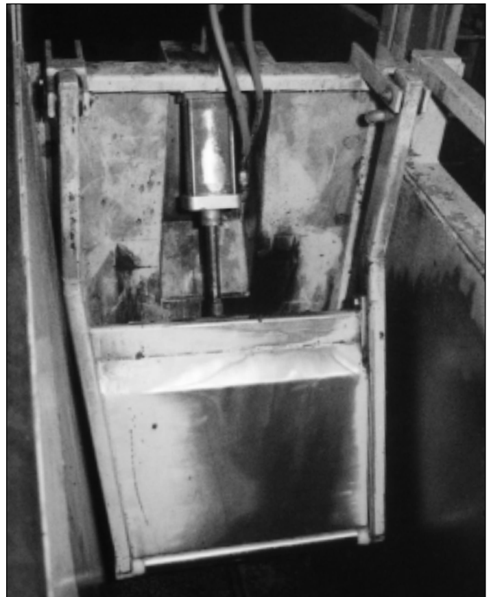
Photograph 1. The pneumatically operated pusher unit in a partially forward position.
